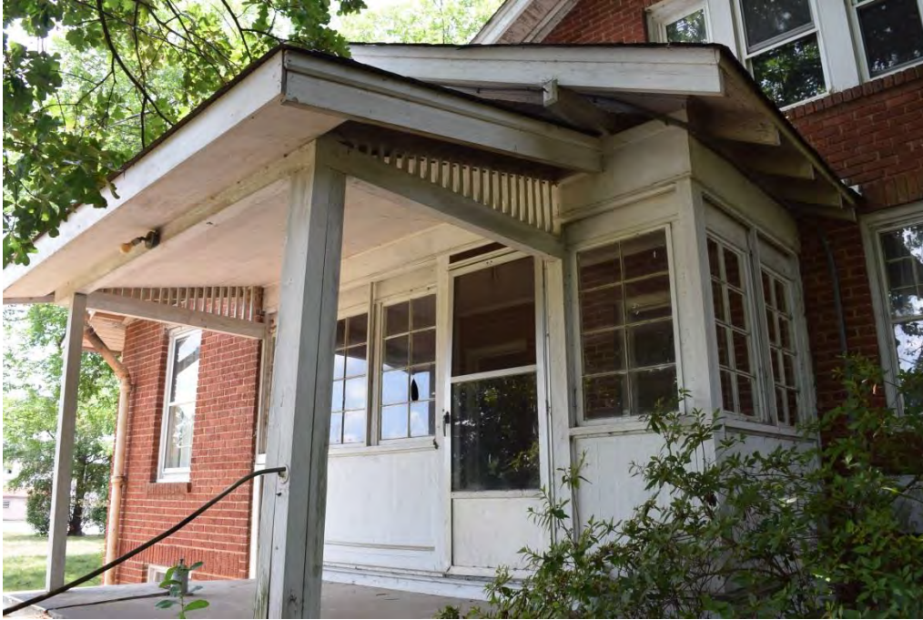
Clonnie Moore House No. 2, Side Wing, Utility Room, and Side Porch, Looking South.
